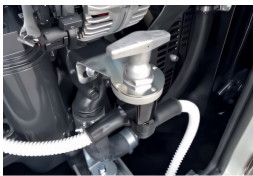
Batterieschalter Battery isolator switch
